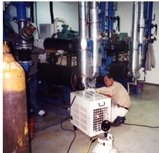
Refrigerant Recovery/recycling process at chiller room in Taiwan.
