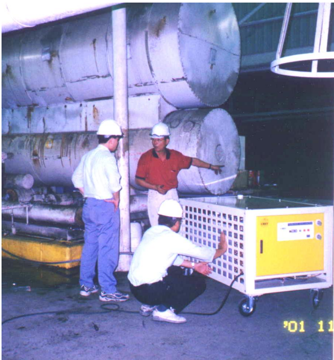
A Recycling and Liquid Refrigerant flushing process for 2000 HP Refrigerator system.
